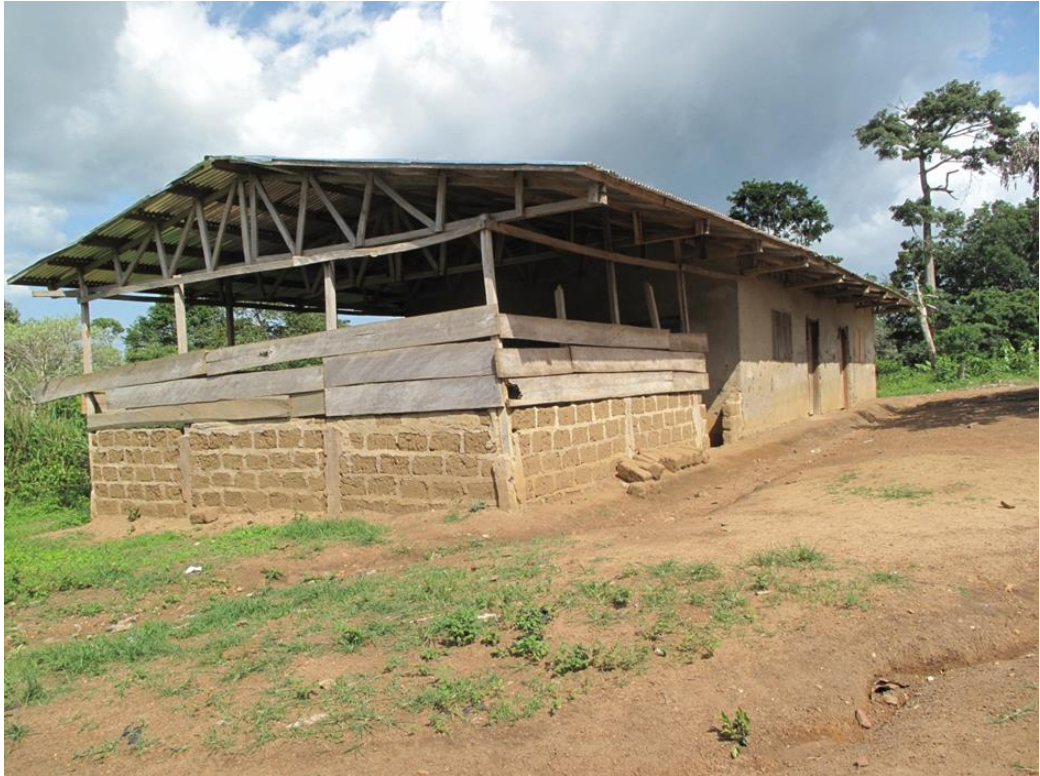
Figure 3: Northern Cape school with a dilapidated building
