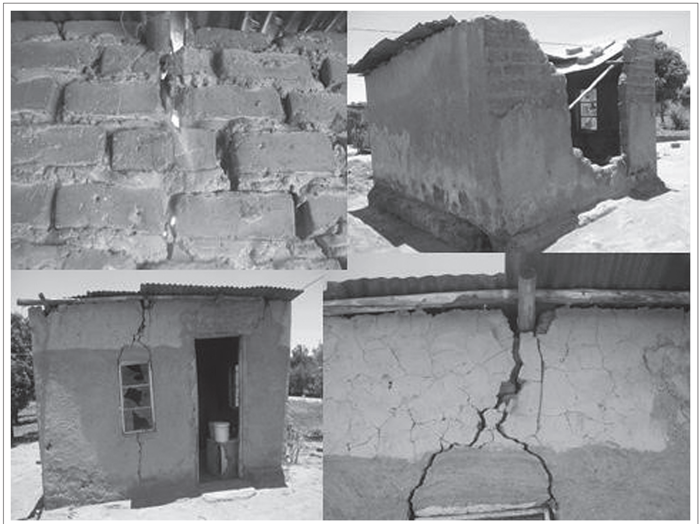
FIGURE 2: Collapsed houses and cracks in Hamutsha-Muongamunwe village.
