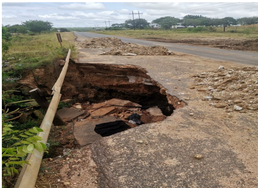
Figure 4: Badly damaged road and bridge at R571 road
