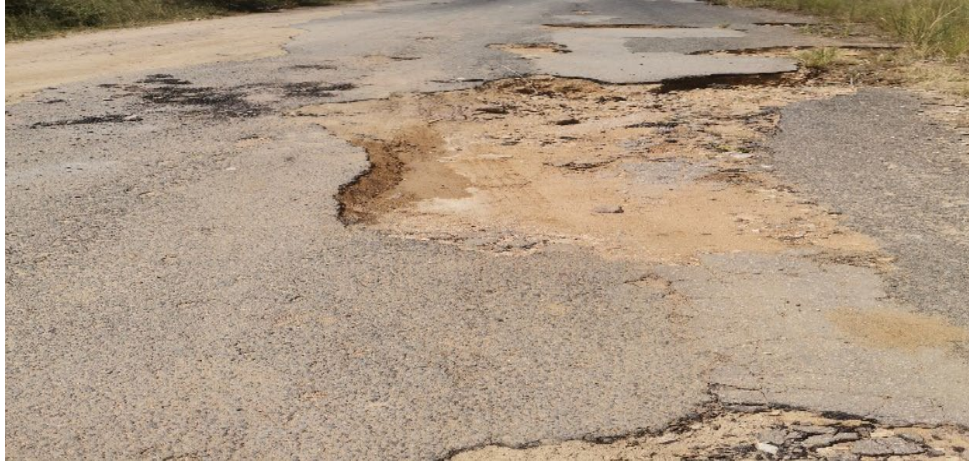
Figure 3: Potholes in R571 road around Nkomazi Local Municipality
