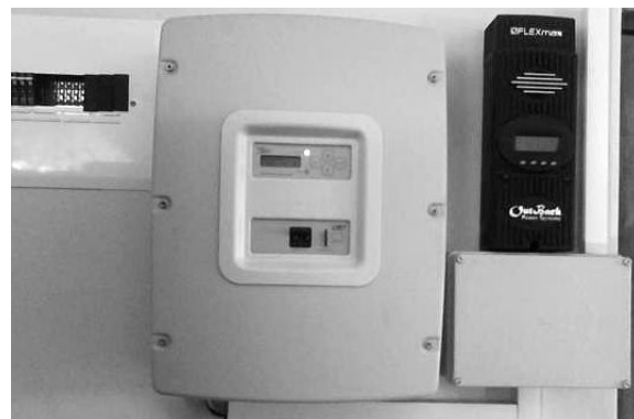
Figure 4: Part of the balance of system components
