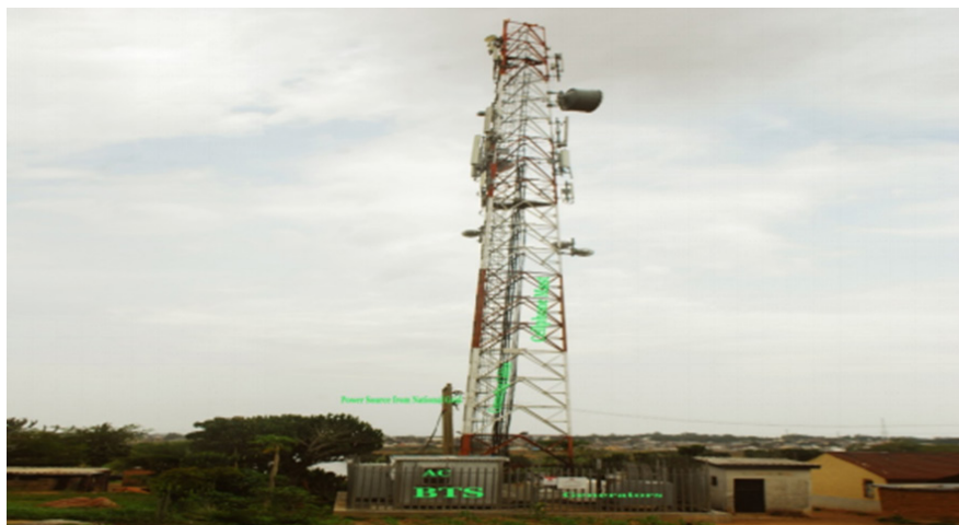
Figure 5. A cell phone base station and some of its components in Via-Fyang, Zawan, Plateau State (Source: EIAR No. 26, 2012, Table 5).
