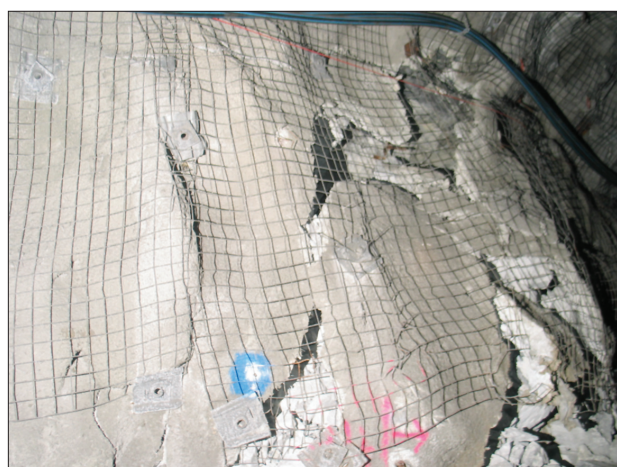
Figure 8—Fibre-reinforced shotcrete cracks due to large deformation and the large plates formed are retained by mesh
