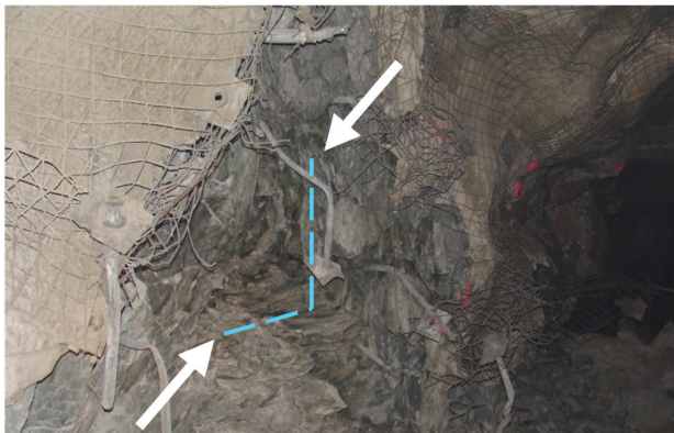
Figure 7—Hanging wall slabs buckling (after DeRoss, 2007)
