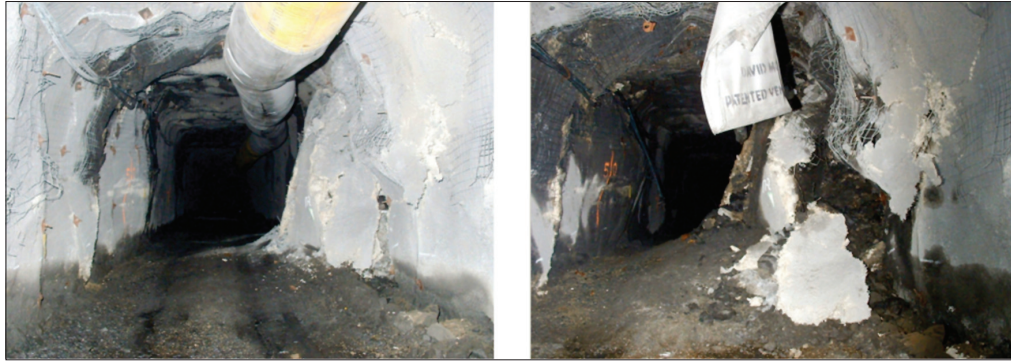
Figure 5—Examples of floor heaving and extensive bulging of the wall: (a) 6 May, 2004 (b) 25 September, 2004
