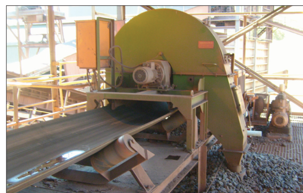
Figure 8—Fully enclosed cross-belt sampler installation
