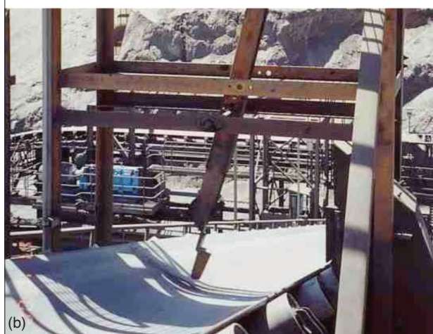
Figure 9—Examples of poorly designed cross-belt cutters. In (a), the conveyor profile does not match the cutter trajectory; in (b) the cutter is simply a paddle
