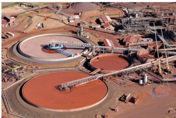
Figure 8—Two by 90 m diameter traction thickeners and common overflow tank
