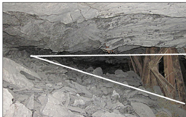
Figure 7 – Example of pillar bursting. The scattered pillar material was ejected into the siding. The white lines indicate the scatter relative to the stope width. Timber elongates indicate dynamic loading as a result of the event
