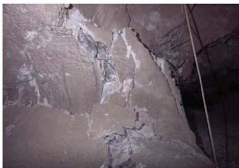
Figure 14—Significant cracking of shotcrete, the installed support system in the main intersection of Copper Cliff's 3200 level, prevented the ejection of broken material on 11 September 2008 (Chinnasane, 2009)
