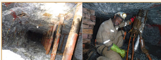
Figure 1—High tensile steel mesh installed in stopes (left – courtesy: Sibanye Stillwater; right – courtesy: Harmony)
