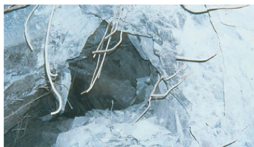
Figure 2—Exposed rockbolts after a rockburst - indications of tension and shear along multiple surfaces (Stacey, 2012)
