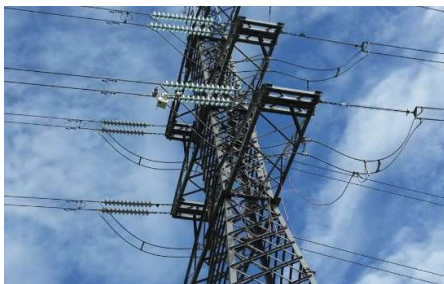
Figure 31 Power line inspection robot climbing from a jumper to the main line on a (220 kV) strain tower.
